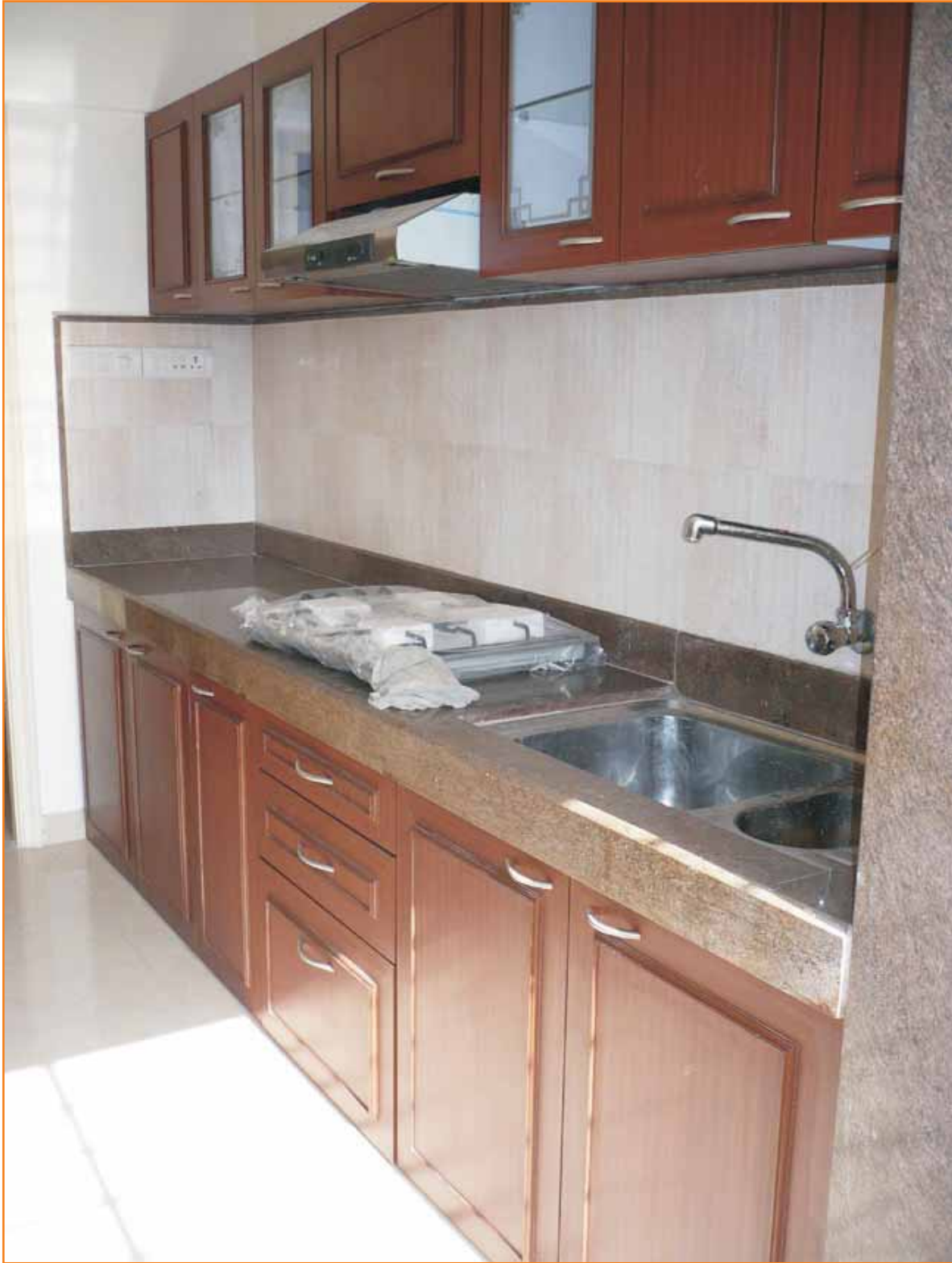
Kitchen service counter
